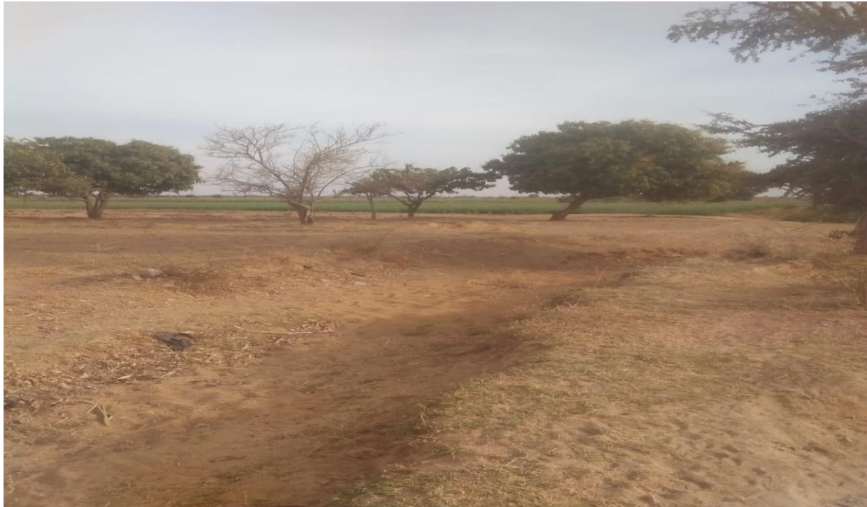
Plate 1: Poor condition of the access road
